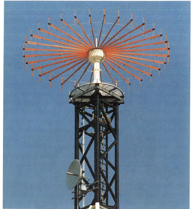
Doppler antenna of one of five VHF Precision Direction Finders PA001 monitoring shipping in the busiest area of the North Sea within the German Bay vessel traffic management system
